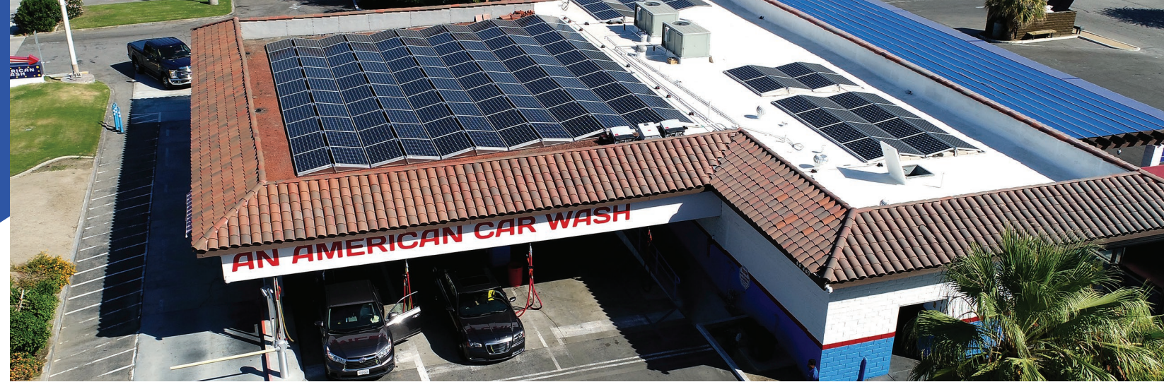
An American Car Wash in Palm Springs, CA. Installation & photo by Renova Energy.
