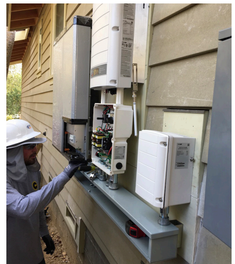
Installing the battery and inverter at a home in California. (Credit: Bernadette Del Chiaro)
