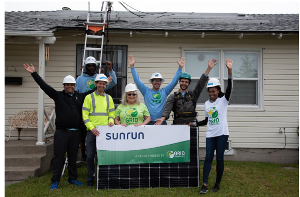
Grid Alternatives and Sunrun partner to build solar roofs for low-income homeowners throughout California as well as provide hands-on experience for workforce training programs. (Credit: Sunrun/Grid Alternatives)
