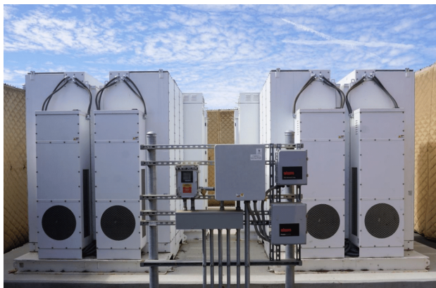
A Stem, Inc. energy storage system. (Credit: Stem, Inc.)
